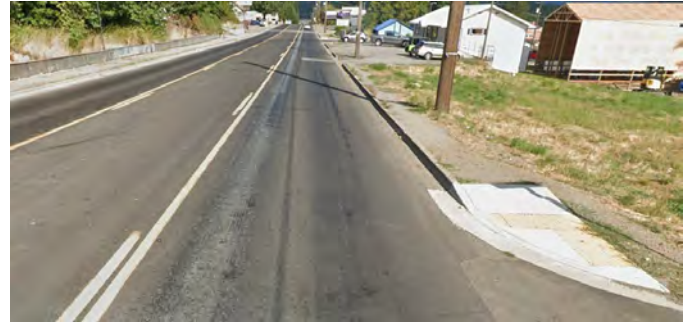
Gaps on US-2 sidewalk.
