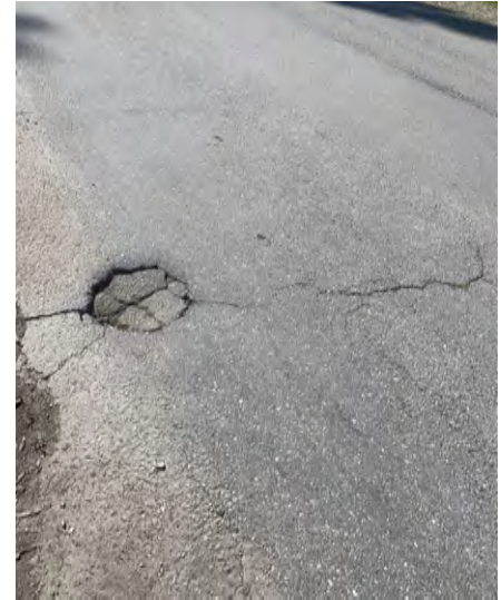
Roadway with potholes that needs maintenance.
